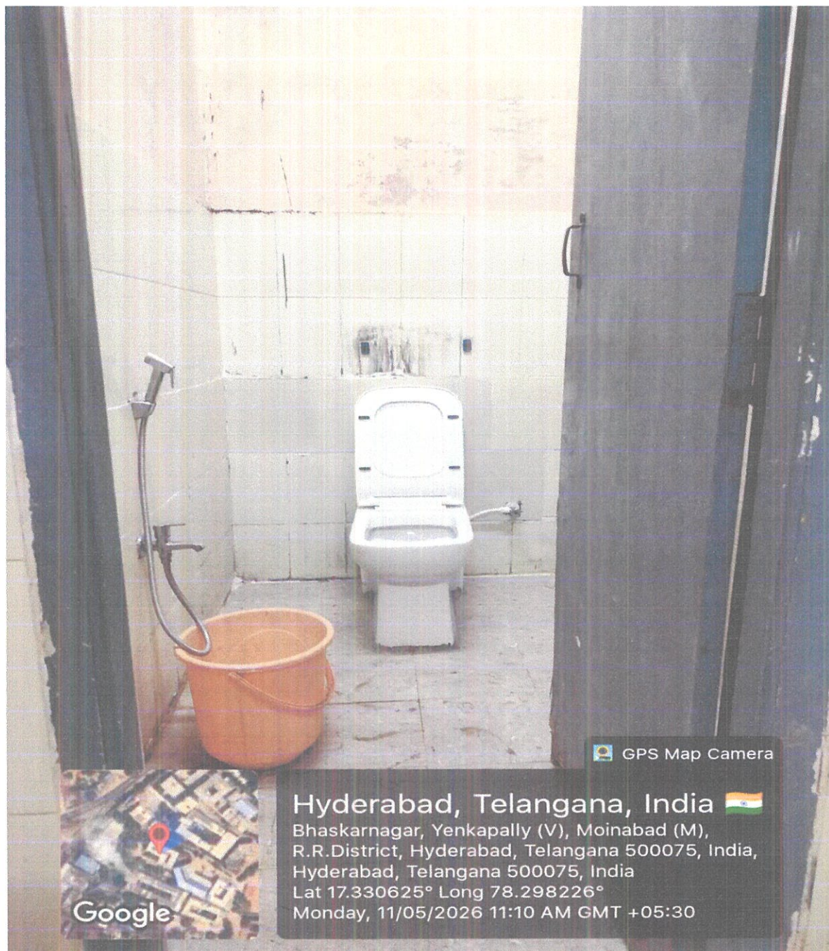
Fig. 8: Disabled Friendly Washrooms
