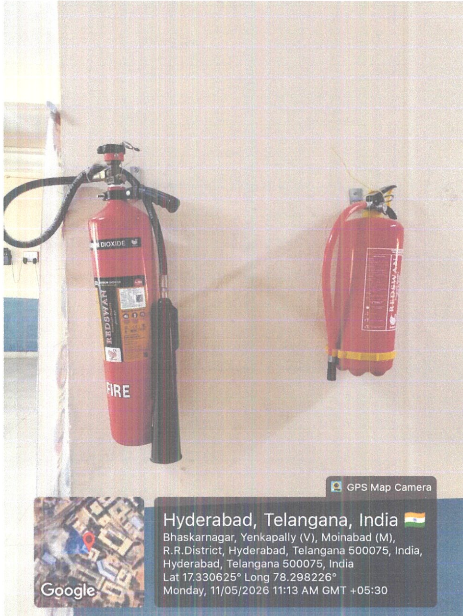
Fig. 14: Sign Board Showing Fire Extinguisher
